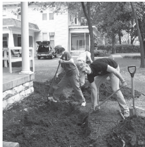
HRWA Staff and volunteers work to install a native rain garden to capture runoff from the parking lot at the office.
