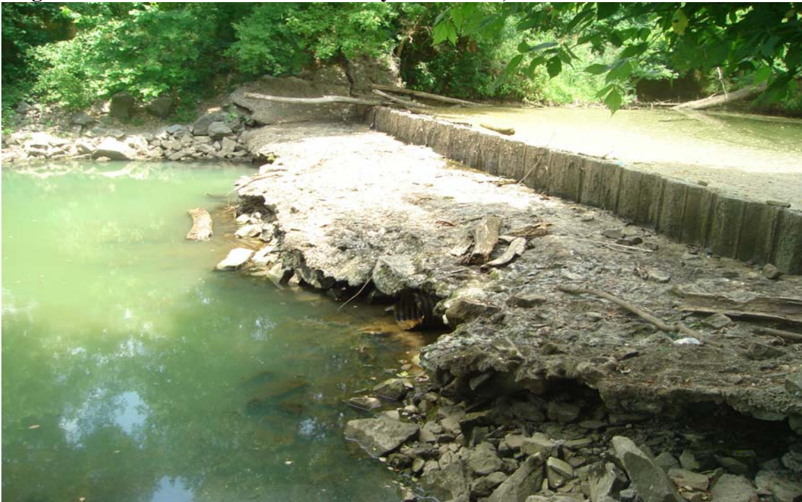
Figure 3: Lowhead dam showing excessive algal growth above water withdrawal.
